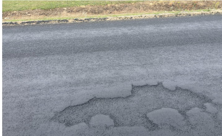
Pictured Below: New Chip Seal with an alligator cracked area that was not patched before paving.
