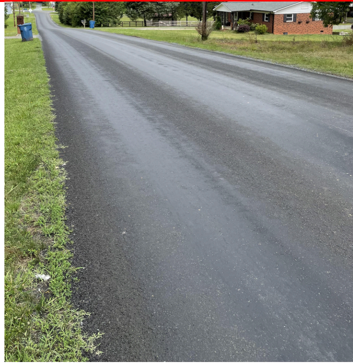
Pictured Above: Bleeding/Flushed Chip Seal, which is worst in the wheelpath, especially under truck traffic.
